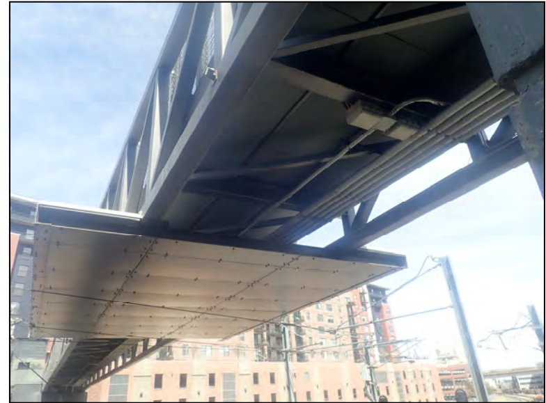
Conduit and Other Attachments Above Light Rail Tracks Looking Northwest
