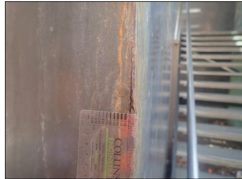
Typical Corrosion at Panel Joints at Stairwell Column Looking East
