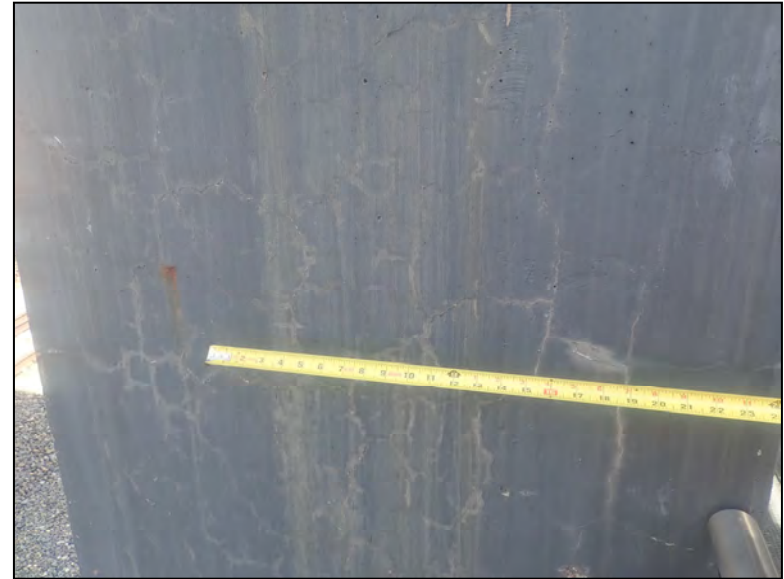
Map Cracking in the South Face of the East Pier Looking North
