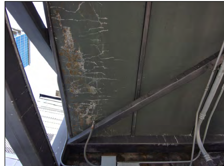
View of Cracking with Efflorescence at Southwest Corner of Underdeck Looking West
