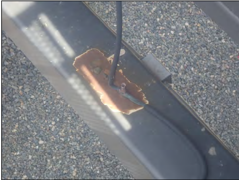
Typical Isolated Area of Corrosion on Lower Chord Looking Northwest
